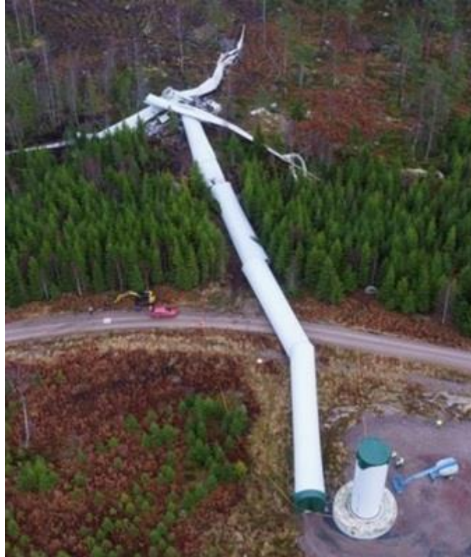
Fig. 1.3 Accident of wind turbine in Lemnhult, Sweden caused by fatigue failure of bolt nut connections.
